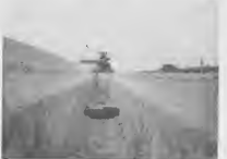
A ditcher opens a neat five-foot trench along the pipeline right-of-way, towing behind a heavy drag to smooth the ditch floor. About 60 per cent of Tappin is buried.
